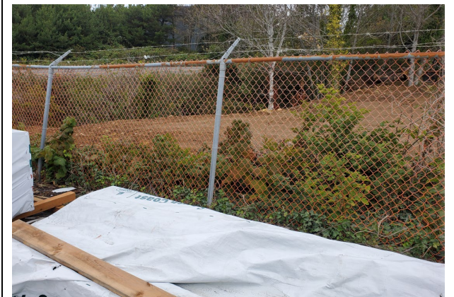
Photo 3: View from the Copeland Lumber Property line. Deep trench in background that has flexible pipe discharging to it
